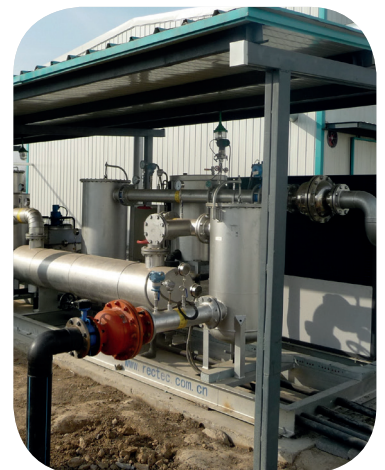
Detail of Luohe's LFG collection and pre-treatment system.
